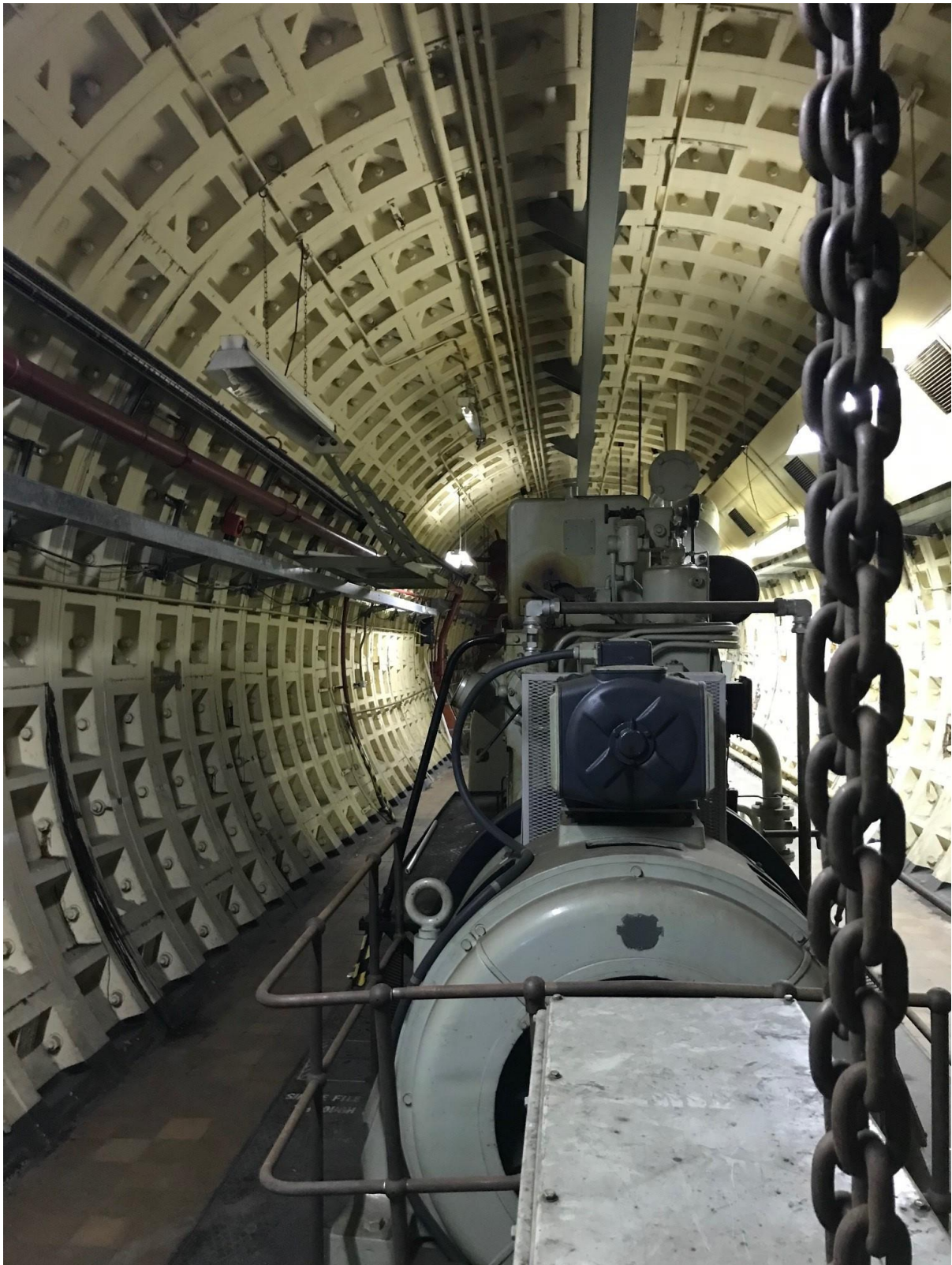
Image 3: Existing equipment with in the Kingsway Tunnels
